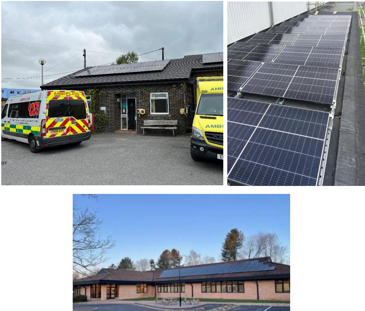
Figure 4: PV installations Lampeter Ambulance Station, Bennett Street and Beacon House 2022-23.
